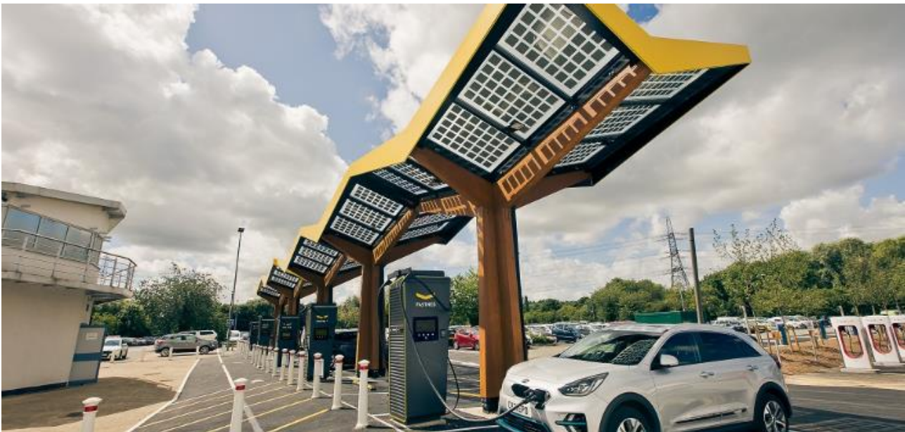
Photo description: Europe’s most powerful EV charging hub in operation at the Redbridge Park and Ride in Oxford.
